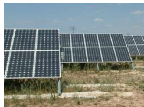
1,5 MW installation (Spain)
